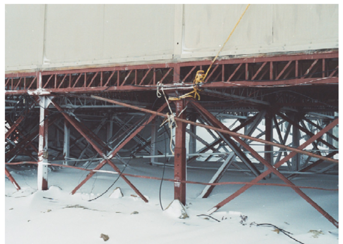
Close-up view of Maitri main block showing steel supporting structure and sandwiched plywood wall panels
