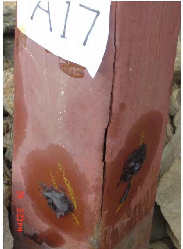
Close-up view of crack in column A17
